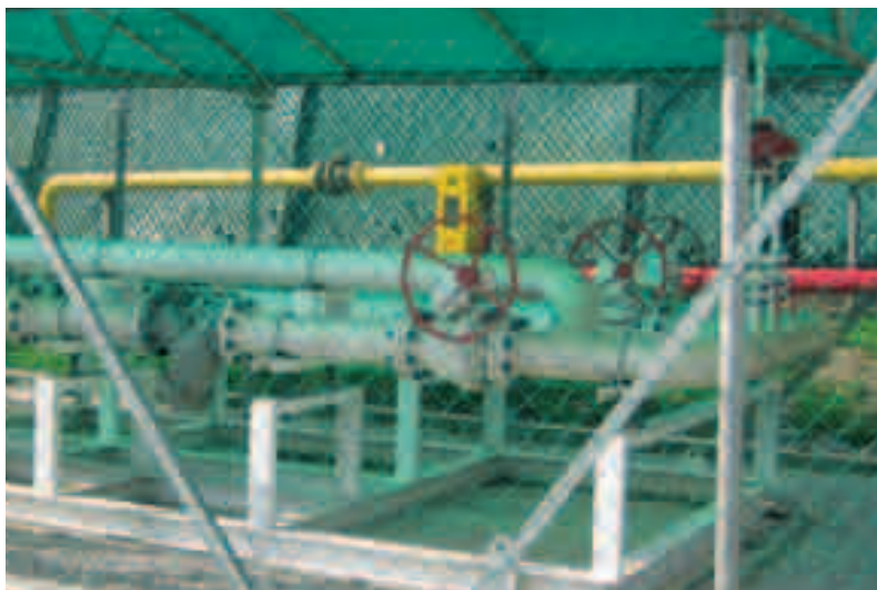
Natural Gas supply station. Stesen pembekal Gas Asli.
