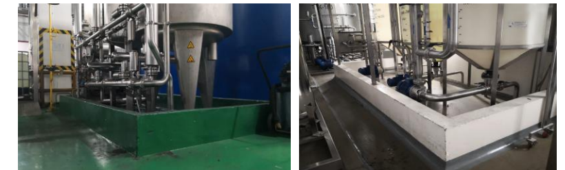
Top row: Raised control panels Bottom row: Brick walls built around the equipment
