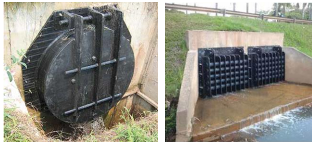
Top: To construct outer bund wall Bottom row: To install flap gates
