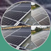
Rooftop Solar PV on cow barns, dormitories, factory and car park
