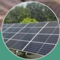
Ground-mounted solar panels
